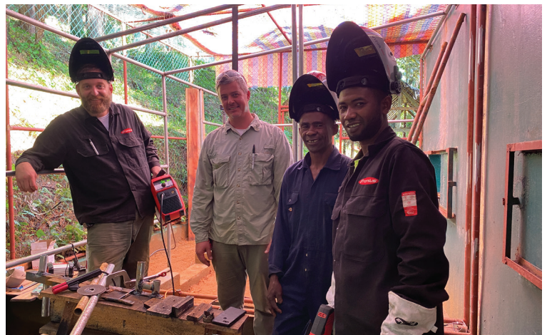
Derek Strunk and Tom Sehnert working with members from the Parc Ivoloina team on the construction of a quarantine space.
