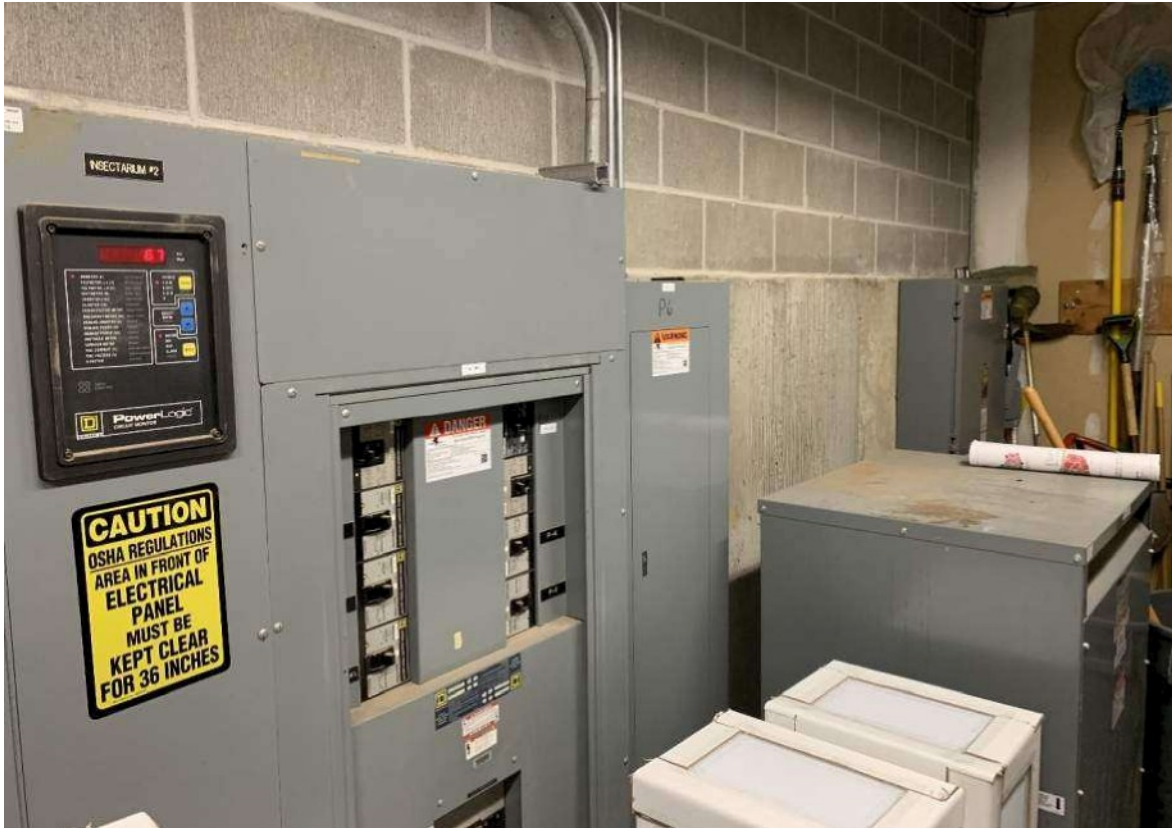
600A MDP in foreground, Panel P6, 225KVA Transformer, and 480V Service Disconnect in Background
