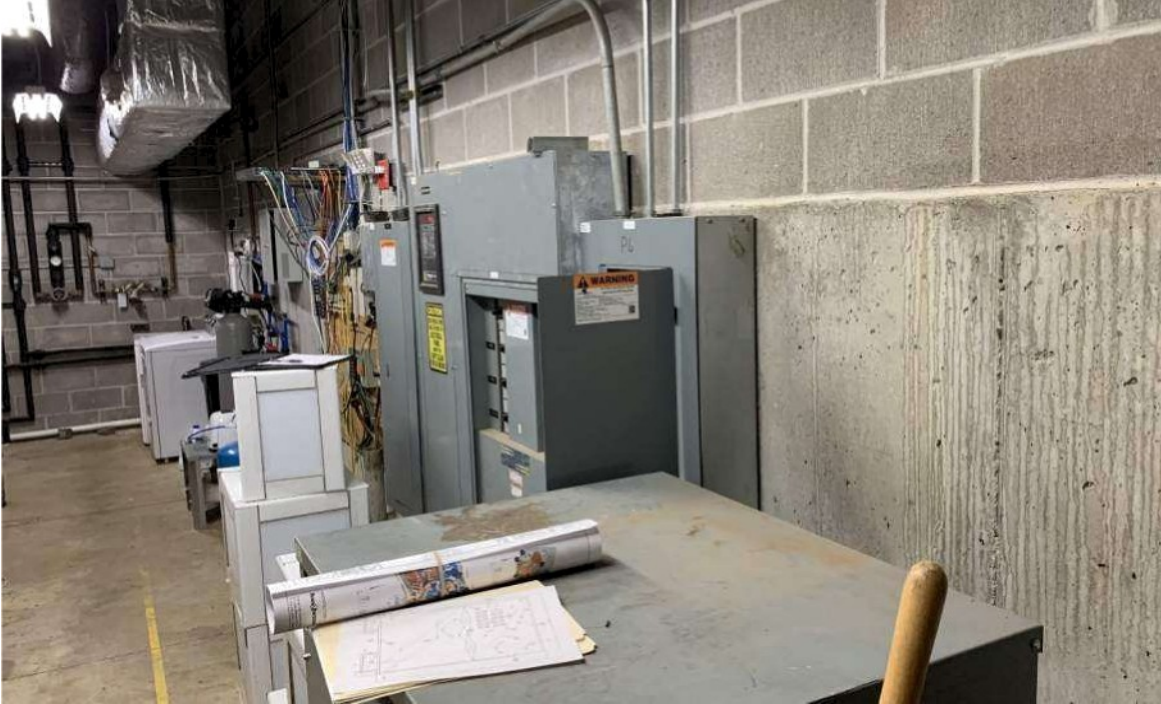
Telecommunications plywood board, Panel P5 to Left of 600A Switchboard MDP, Panel P6 to right
