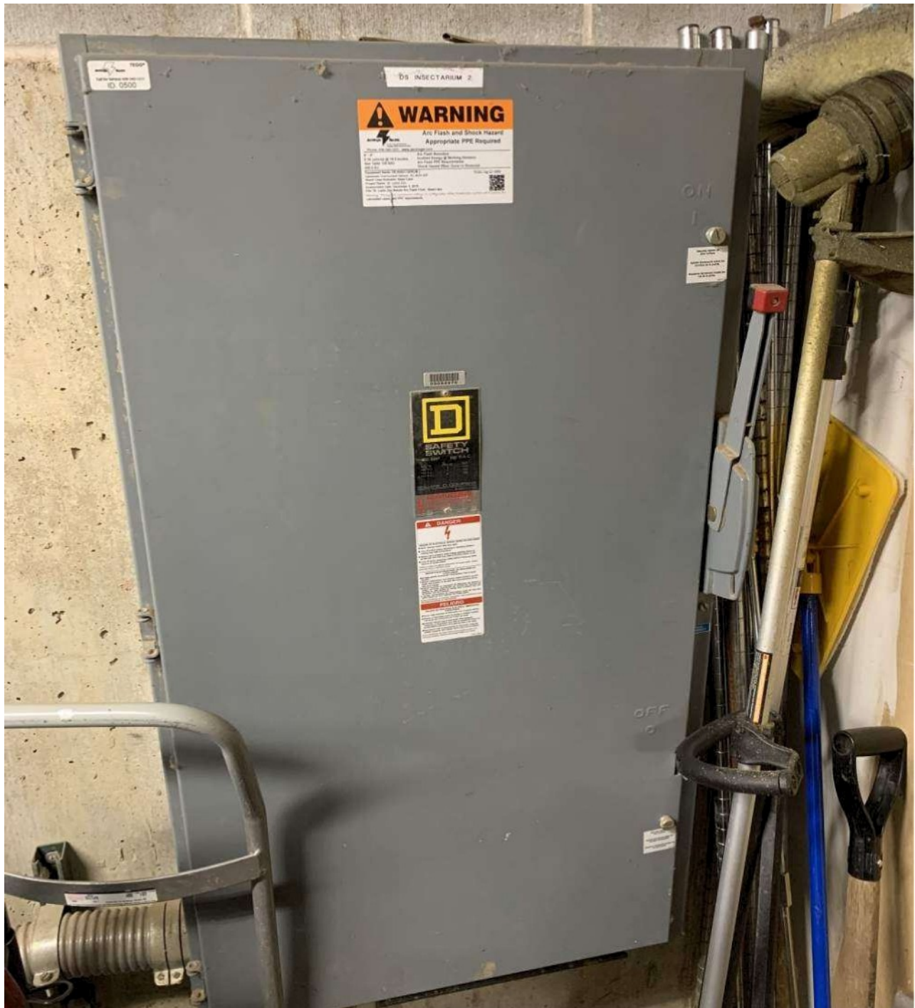
400A, 480V, 3PH SERVICE DISCONNECT
