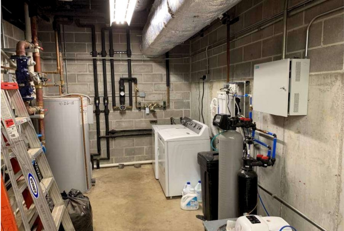
Control Panel, Washer/Dryer and other infrastructure in back area of Storage Room
